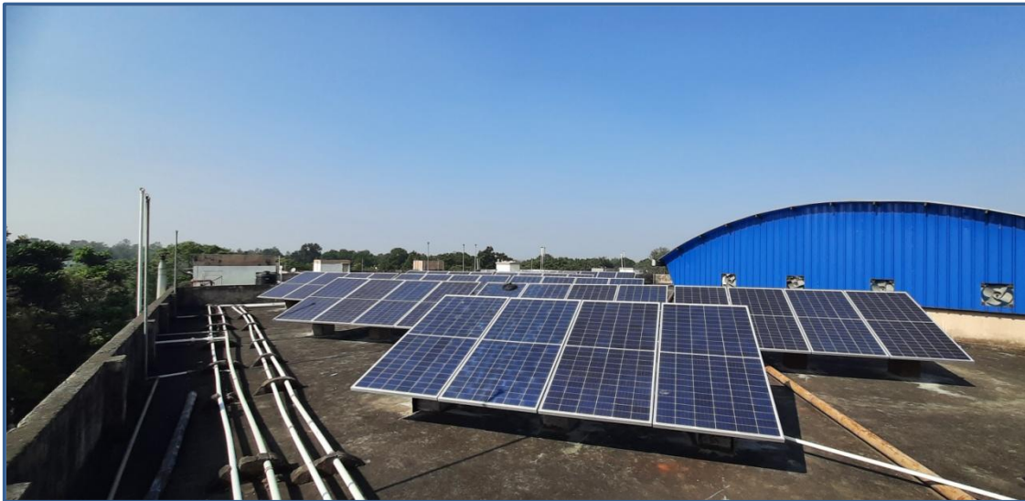
15 kW On-Grid Rooftop Solar Panel
